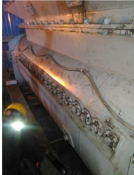
Figure 3.3 Coal Feeder of the Teluk Sirih PLTU
