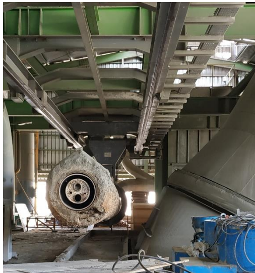
Figure 2.9 Burner (Personal Documentation Resources)
