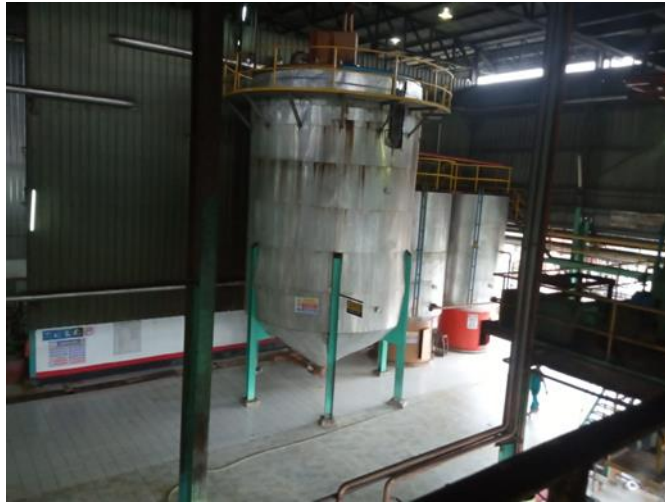
Figure 2.9 Clarification Station (Purification Station)
